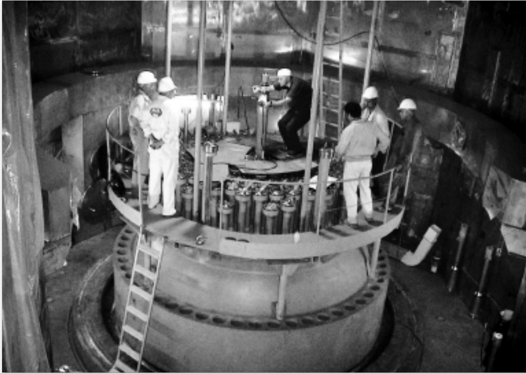
A 2004 view of Russian workers aiding the construction of the Bushehr nuclear power plant in southern Iran.
